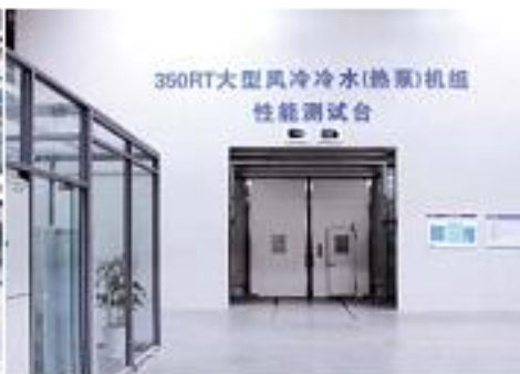
350RT Air-cooled Chiller Test Lab
