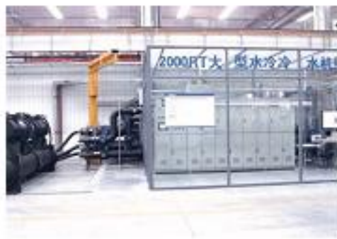
2000RT Water-cooled Chiller Test Lab
